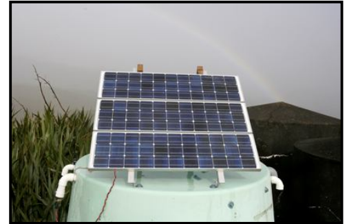
Photovoltaic panels for harnessing sun power
